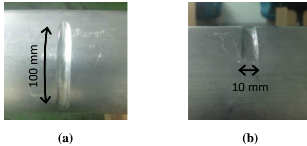
Figure 3: Circumferential defect of 3 mm depth in the pipe: (a) Top view (b) Side view.
