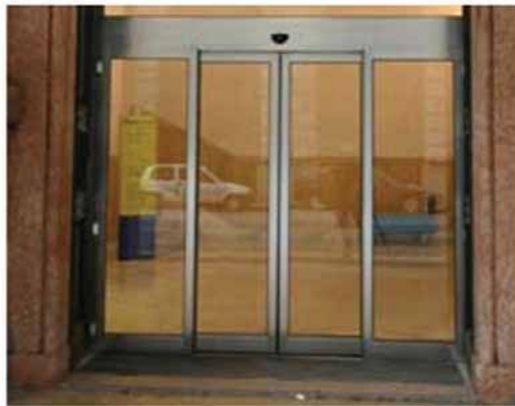
Figure 6: Example of emergency door with reinforced glass.
