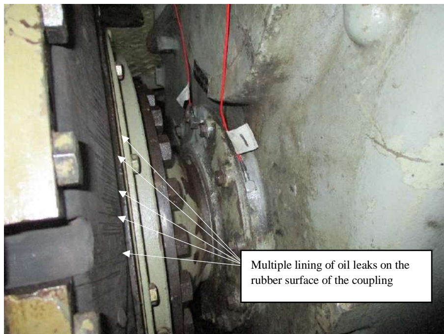
Figure 1: The damaged flexible coupling investigated in this study.
